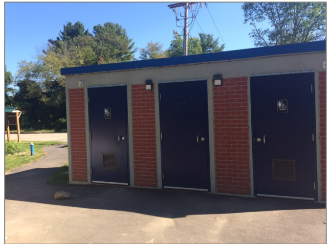
Handicapped accessible bathrooms. Bathrooms were locked at the time of site visit and are assumed to meet ADA standards because of the signs on the doors.
